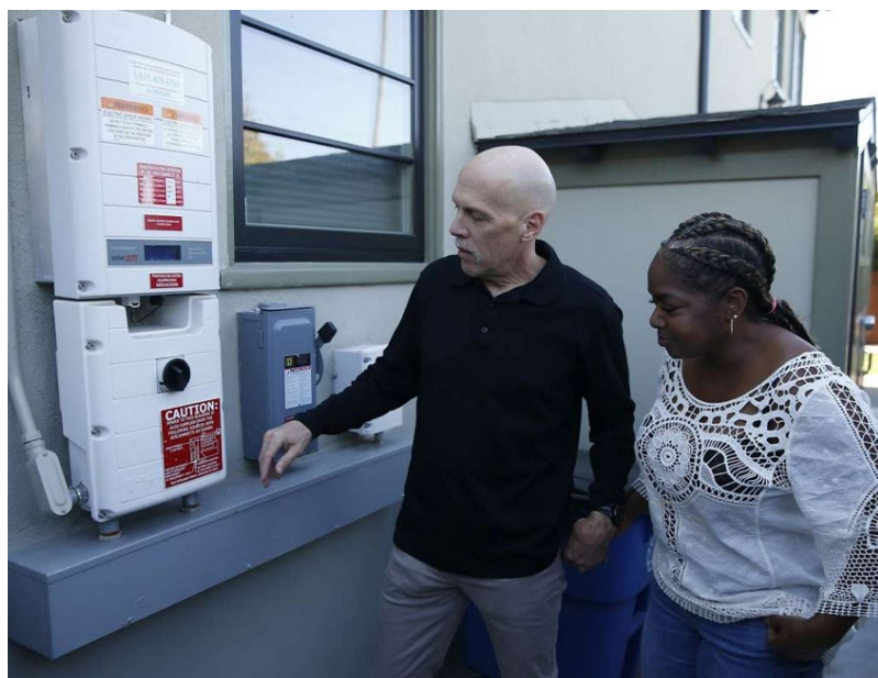
Derek and Dorothy Krause check the utility panel for the solar energy and backup system installed at their home in Oakland, Calif. on Tuesday, Oct. 22, 2019. Source: Paul Chinn, San Francisco Chronicle
