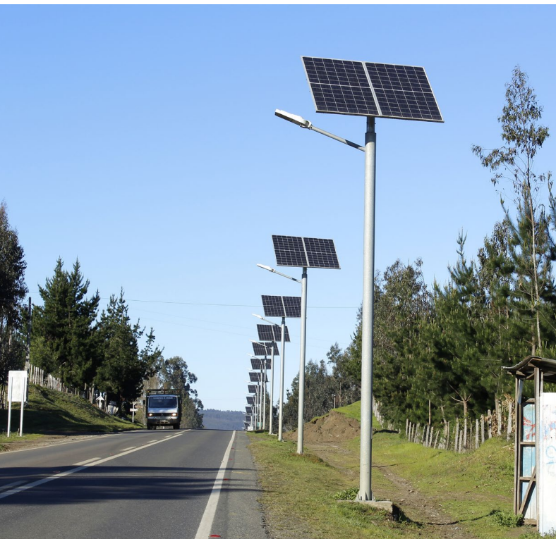
Solar street lights
